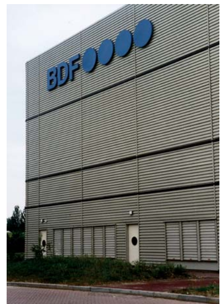
Seefire natural louvred ventilators installed at low level.
