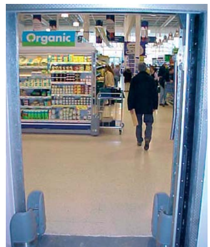
Colt Firepath fire curtains installed at Tesco's in Glasgow. These are designed to separate the main shopping area from the storage area.
