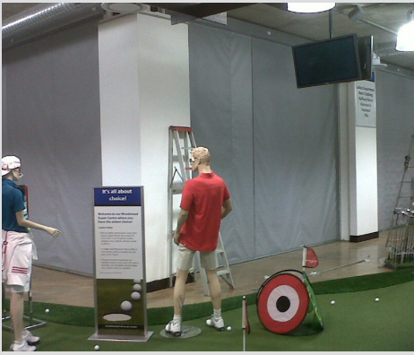
Retail - fire curtain lowered
