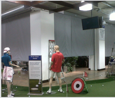
Retail - fire curtain in mid position
