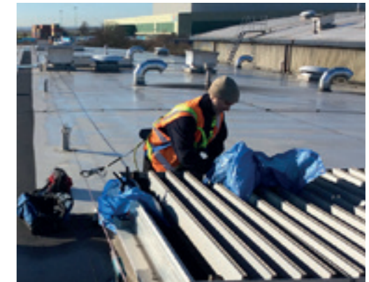
Whether built by us or others, all smoke and climate control systems can be expertly maintained by our engineers.
